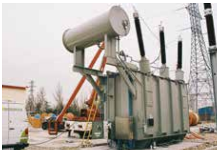
Figure 2. Baseline field testing of a power transformer before going into service (50 MVA)
