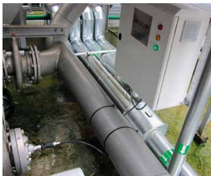
b) Monitoring system with UHF sensor
