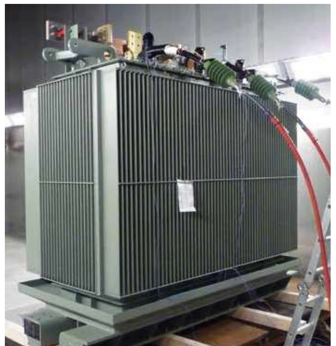
Figure 8: 5.56 MVA Bio-SLIM transformer inside the climatic chamber at -30 °C
