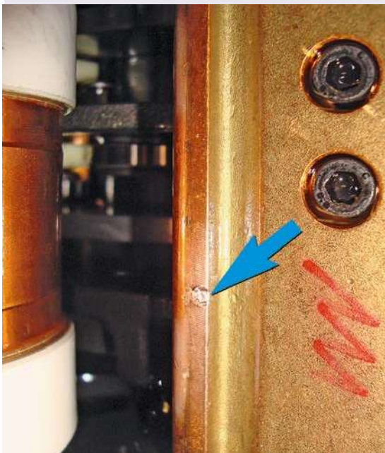
Figure 2. Arcing mark of a low-energy flash-over on OLTC main contact, caused by an overvoltage surge
