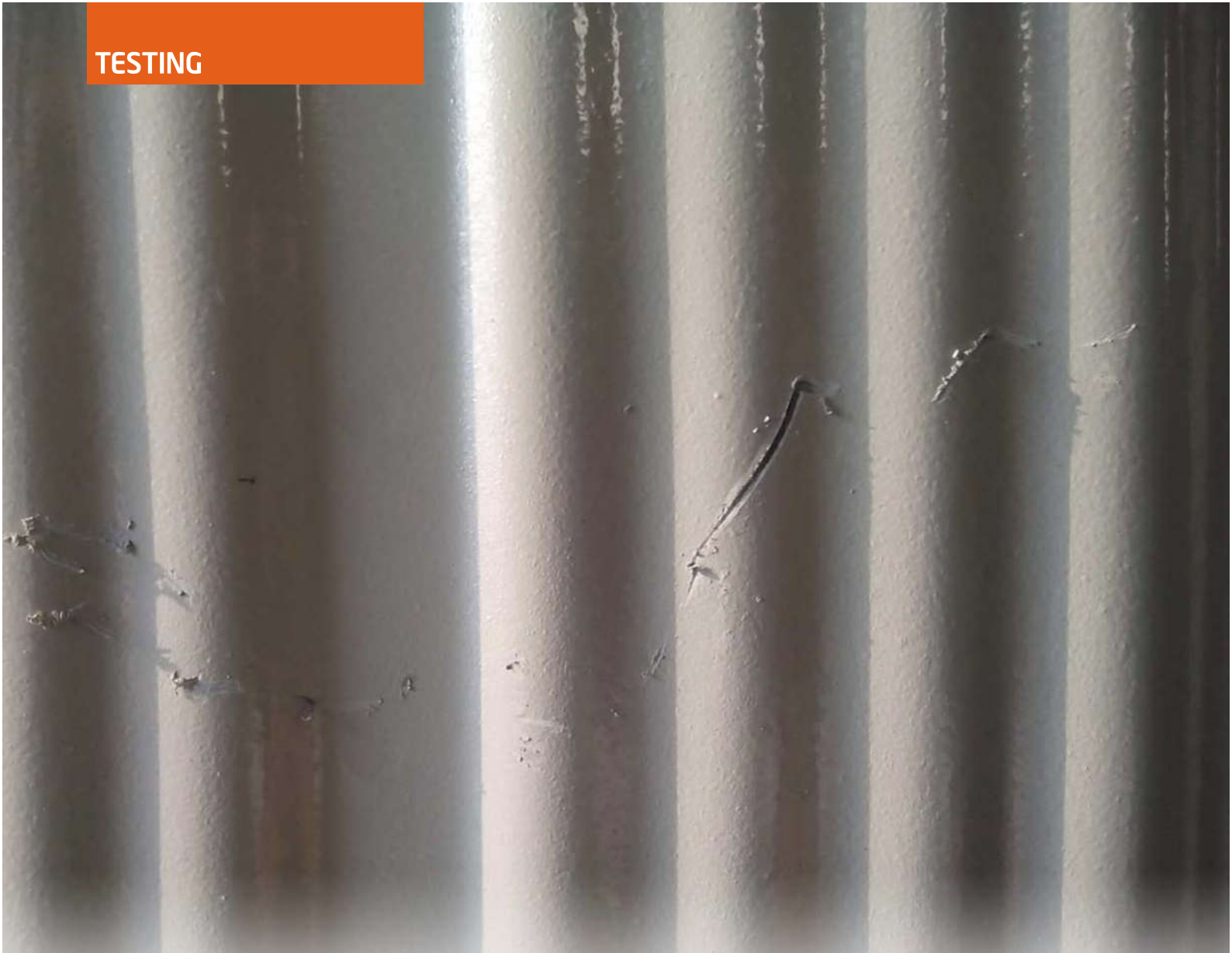
Figure 1. Scratches in the protective surface coating of a transformer tank
