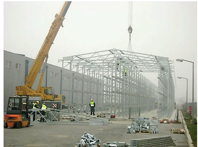
Figure 9 Assembling and installation of roof truss made of open rack column section
