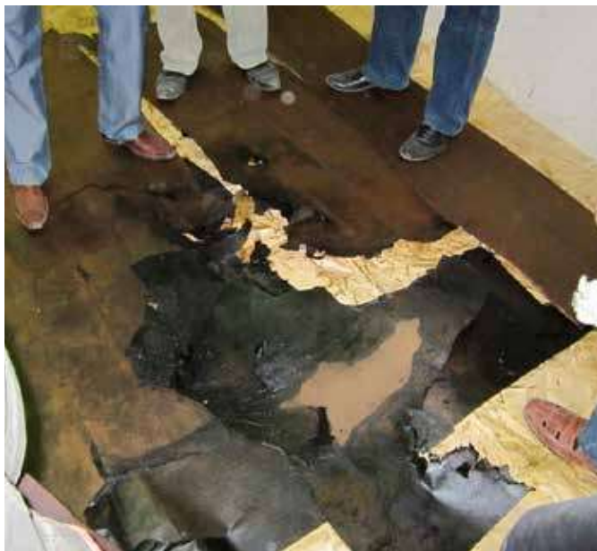
Figure 2: Burnt cardboard insulation
