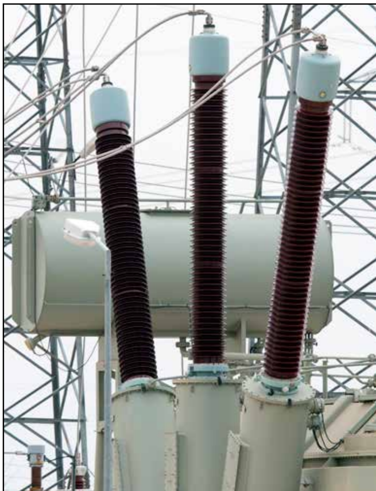
Figure 3: High voltage bushings of power transformer
