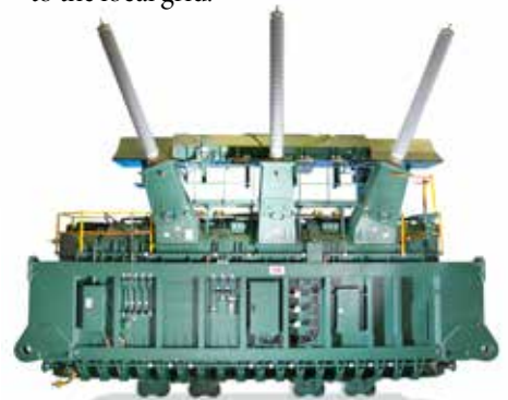
Figure 4: GSU transformer 890 MVA [4]
