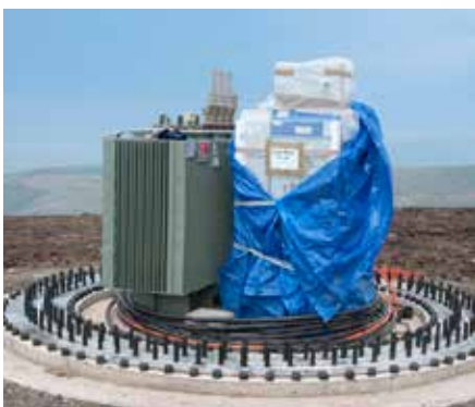
Figure 18: Wind turbine transformer [8]
