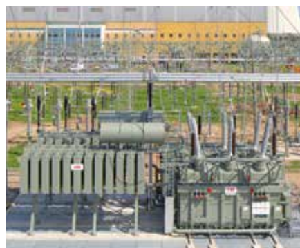
Figure 6: PST 600 MVA, 230 kV [4]
