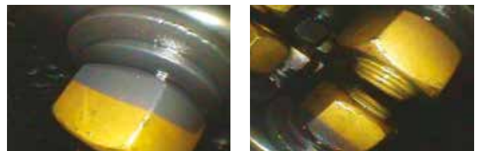
Figure 10: Typical contaminated bolt from a GSUB transformer affected by sulfur corrosion
