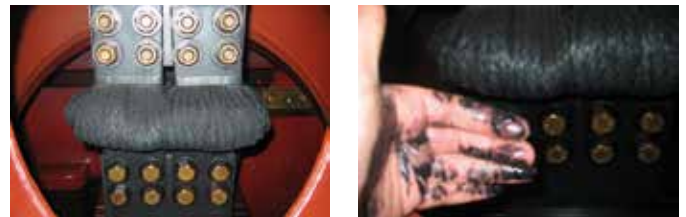
Figure 9: LV side (10.5 KV) flexible connection from a GSUB transformer affected by sulfur corrosion
