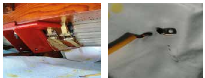
Figure 4. Case 1 Transmission transformer, DGA + findings
