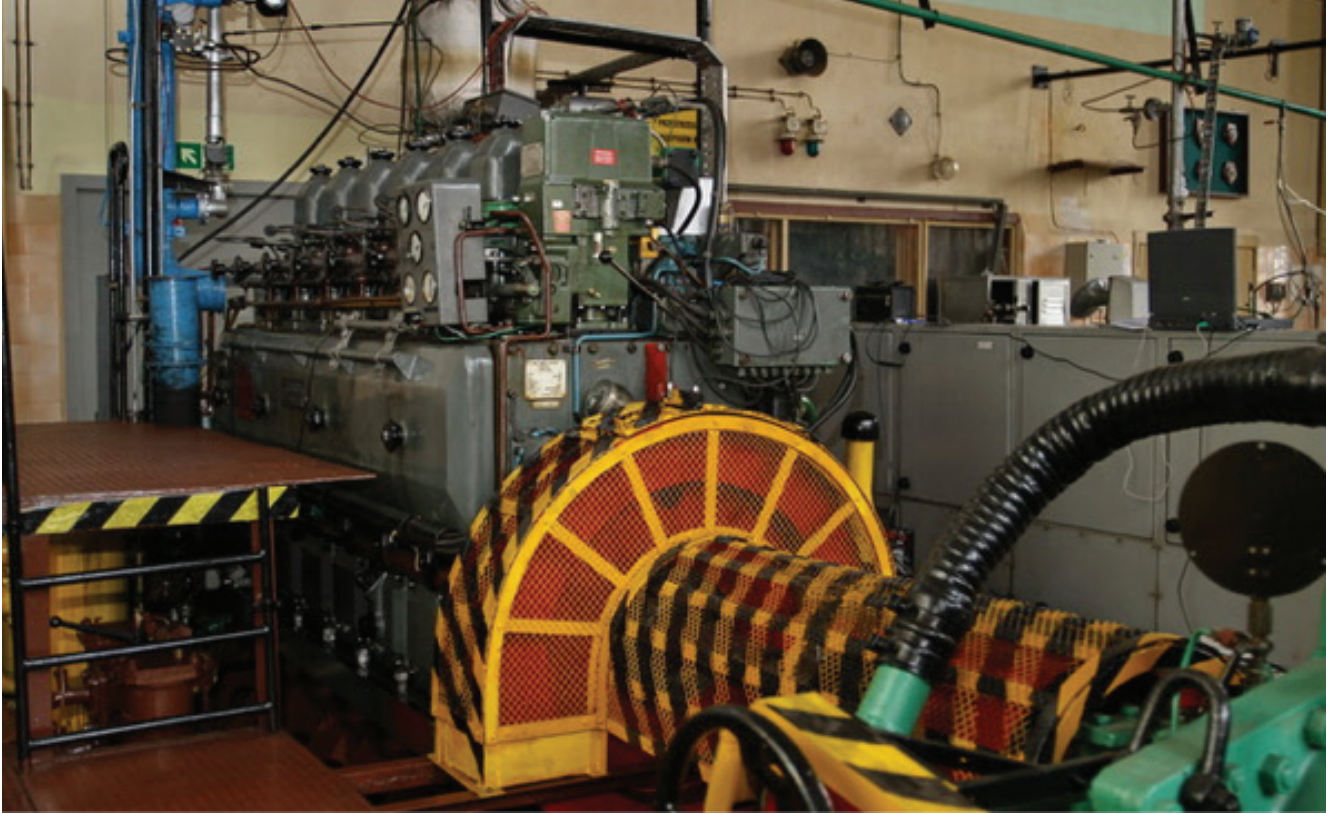
Figure 1. Sulzer 8AL 25/30 type engine test stand in the Laboratory of the Faculty of Mechanical & Electrical Engineering of the Polish Naval Academy.
