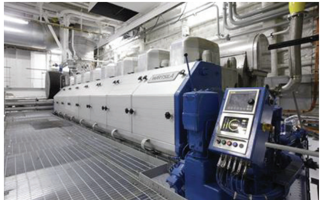
Figure 1. Engines inside Viking Grace's engine room.
