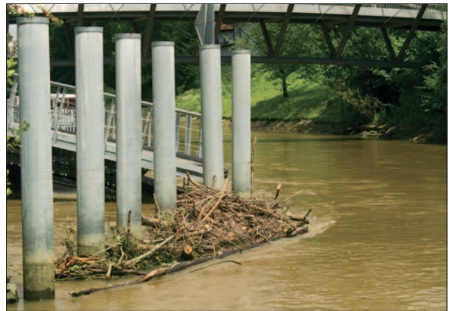
Fig. 11 The accumulation of organic material at the metallic piles of the riverine port at Špica in Ljubljana (photo: D. Valoh)
