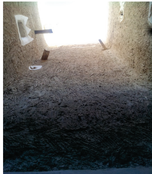
Figure 10 Openings in the ceiling alleys for air circulation
