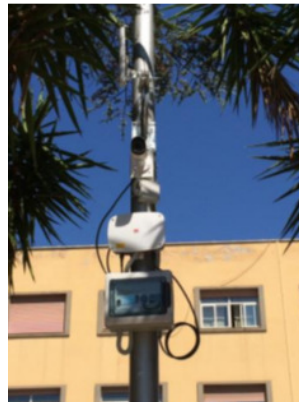
Figure 4. Pole with additional devices
