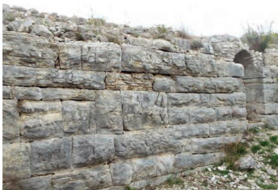
Sl. 38. Vanjsko lice bedema uz nadsvođeni prolaz – pogled na manje razlike u zidnoj strukturi Fig. 38. Outer face of wall next to arched passage – view of minor variations in wall structure (foto / photo by: B. Štefanac)
