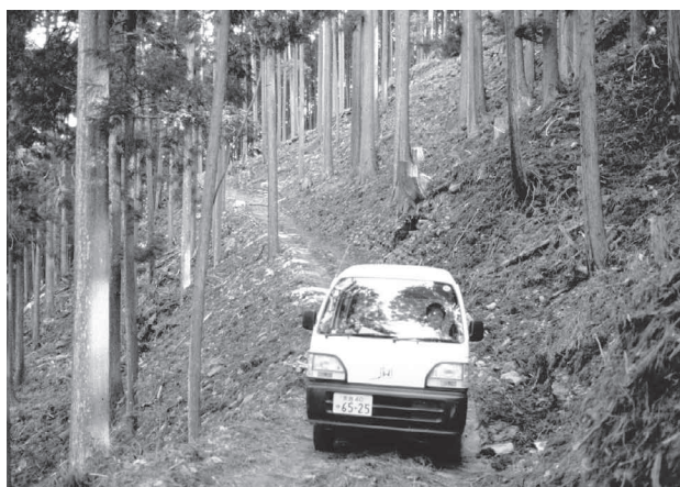
Fig. 8 Road constructed by retaining wall with log structure with narrow width of 2.5 m and a light truck
