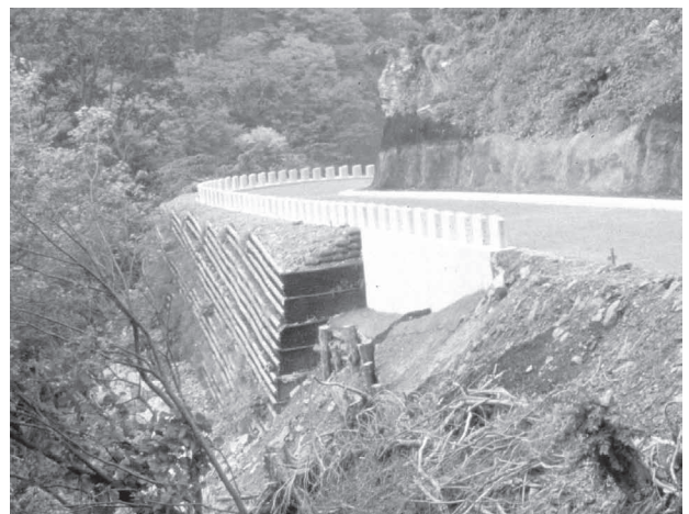
Fig. 21 A reinforced soil wall, TK wall, applied at the site where the height of the filling exceeded 2 m
