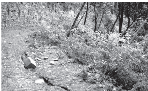
Fig. 18 Filling and constructing the retaining wall is impossible at the ridge when crashing zone and dip slope overlap
