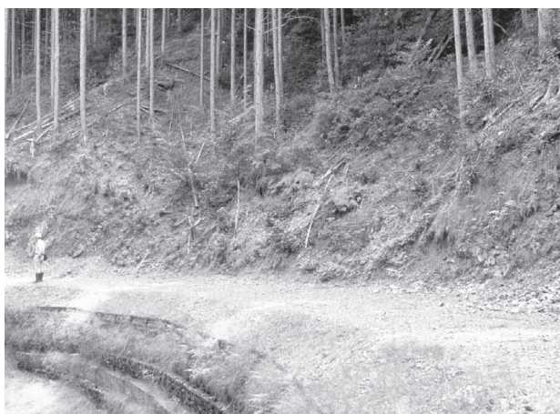
Fig. 22 Retaining wall whose surface was covered by vegetation, L-shaped steel retaining wall, set on three cages stacked on top of each other when crossing a crushing zone
