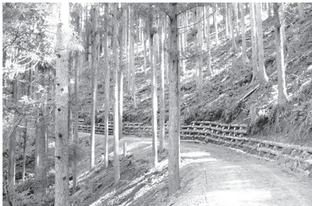
Fig. 12 Retaining wall with log structure is effective for deposit of debris flow
