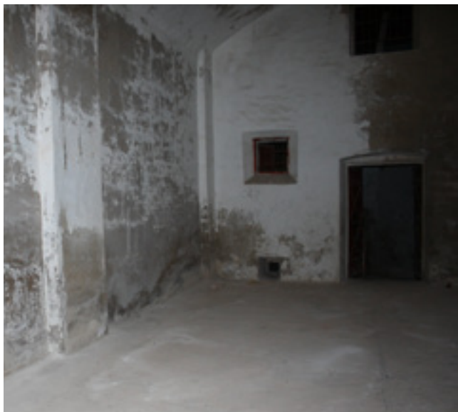
14. Lezene u unutrašnjosti barutane u tvrđavi sv. Nikole (foto: I. Glavaš) Pilaster strips in the interior of the gunpowder magazine in St Nicholas' fort
