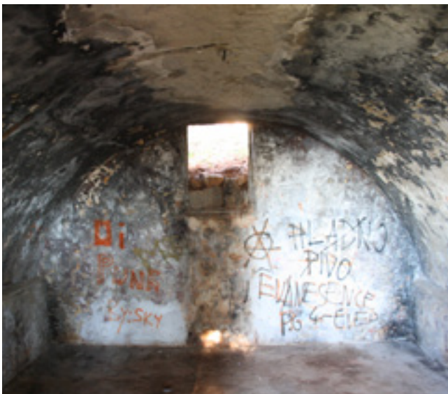
21. Unutrašnjost barutane na tvrđavi sv. Ivana (foto: I. Glavaš) Interior of the gunpowder magazine in St John's fort
