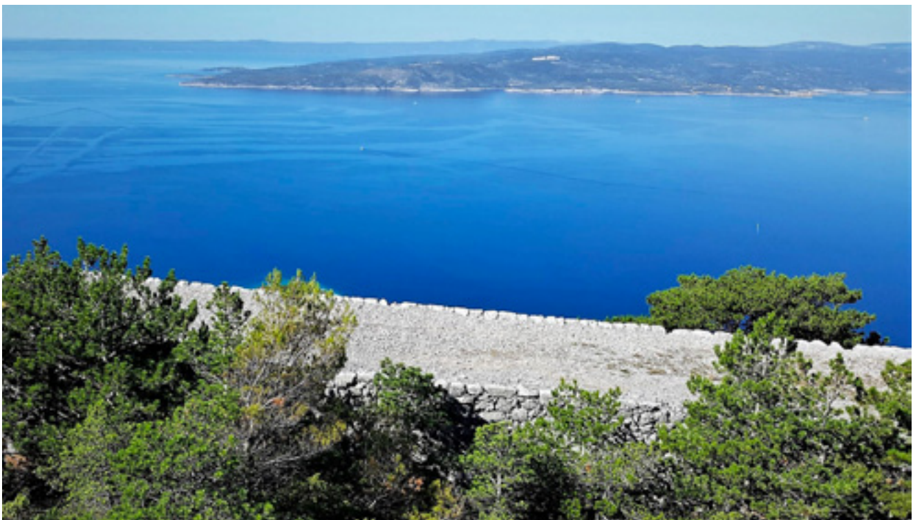
8. Dijelovi trase kolnika teku izdignuti nad terenom. Niski podzid s vertikalnim vanjskim licem Parts of the road are raised above the terrain; a low retaining wall with a vertical mantle
