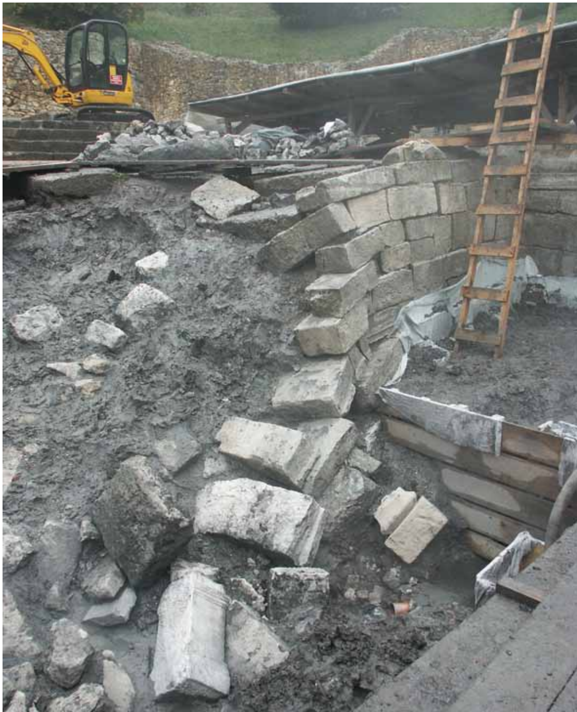
Slika / Figure 8: Pogled na urušeni sjeverni zid izvorišnog bazena, tijekom istraživanja 2011. god. (snimila D. Nemeth-Ehrlich). / A collapsed northern wall of the spring reservoir during the 2011 excavations (photo by D. Nemeth-Ehrlich).
