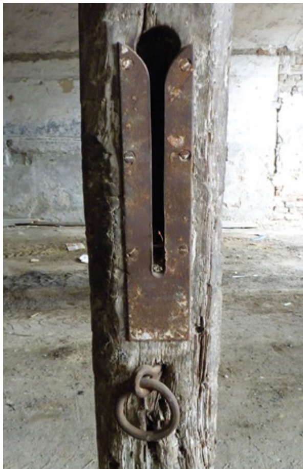
15. Metalni utori na drvenim stupovima konjušnice za ugradnju pregrada (fototeka HRZ-a, snimila I. Pauk Sili) Metal slots for installing partitions on wooden columns in the stables (Croatian Conservation Institute Photo Archive, photo by I. Pauk Sili)
