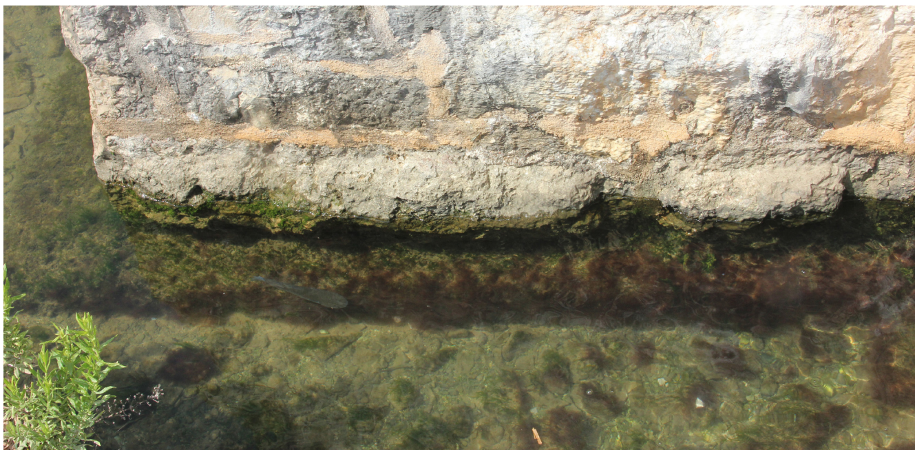
Sl. 2. Podnožje kontrafora s južne strane Mlinice (kontrafor lijevo od ulaza u kulu) Fig. 2. Foot of the counterfort on the southern side of Mlinica (counterfort left of the entrance to the tower)
