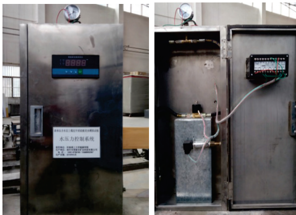
(a) Outside (b) Inside Figure 2 Intelligent water pressure controller
