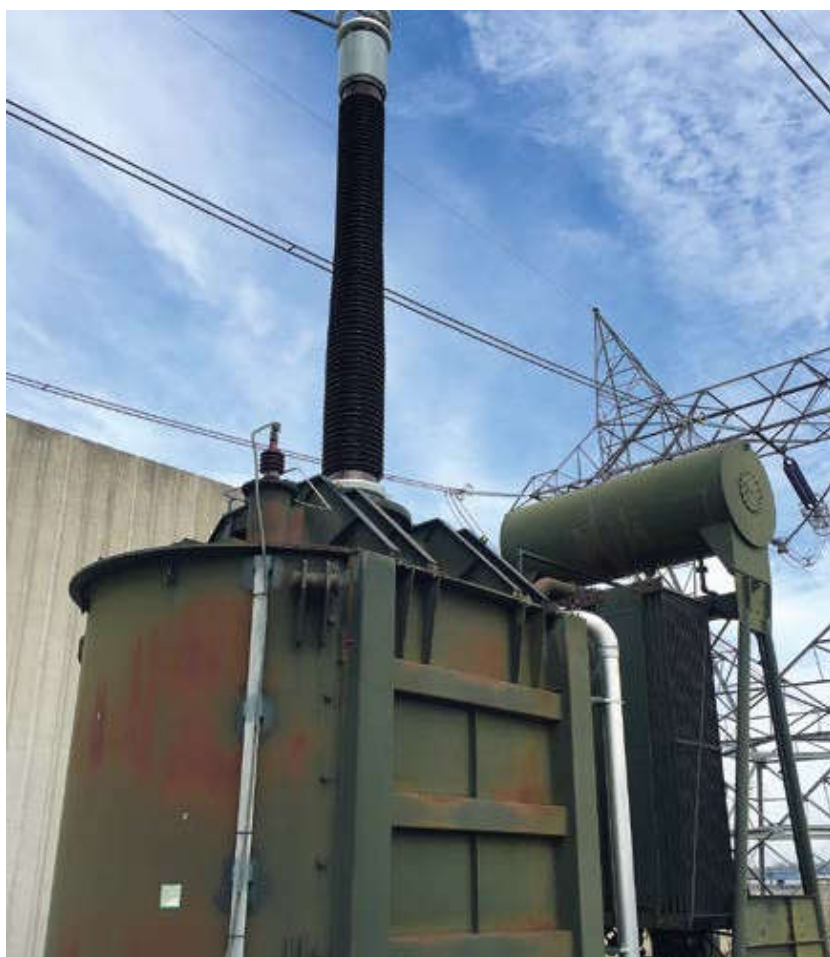
Figure 3. Shunt reactor with EHV OIP bushing
