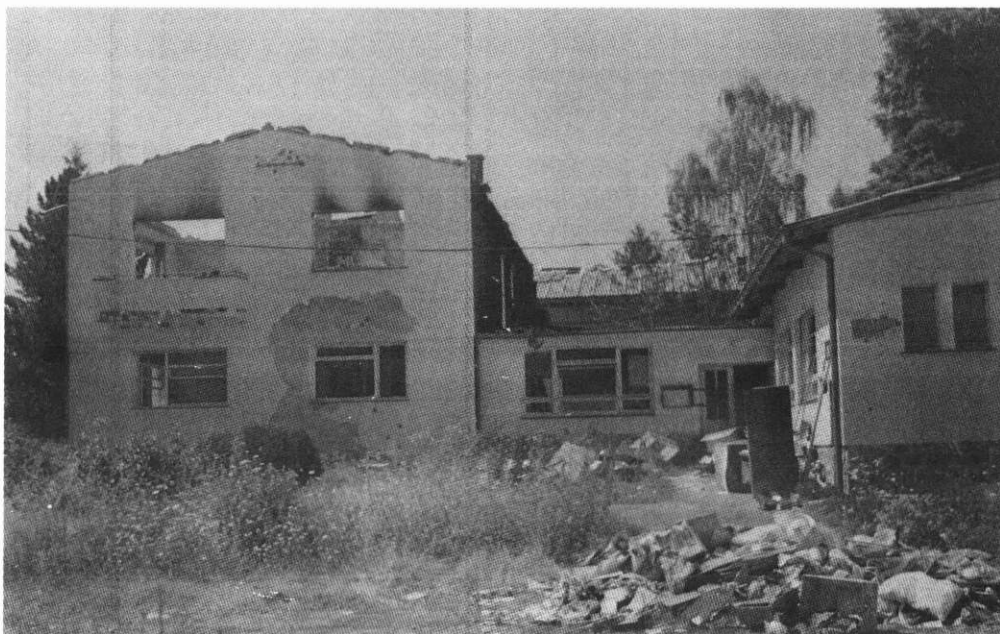
SLIKA 1. Razrušena područna ambulanta u selu Voćinu FIGURE 1. Demolished district outpatient in the village of Voćin
