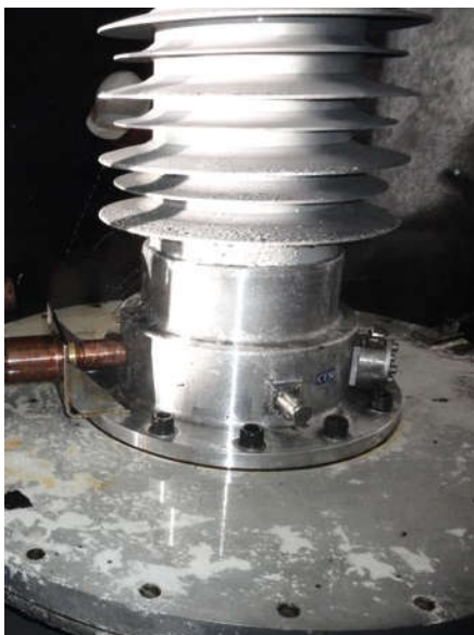
Figure 9. OIP bushing after the test
