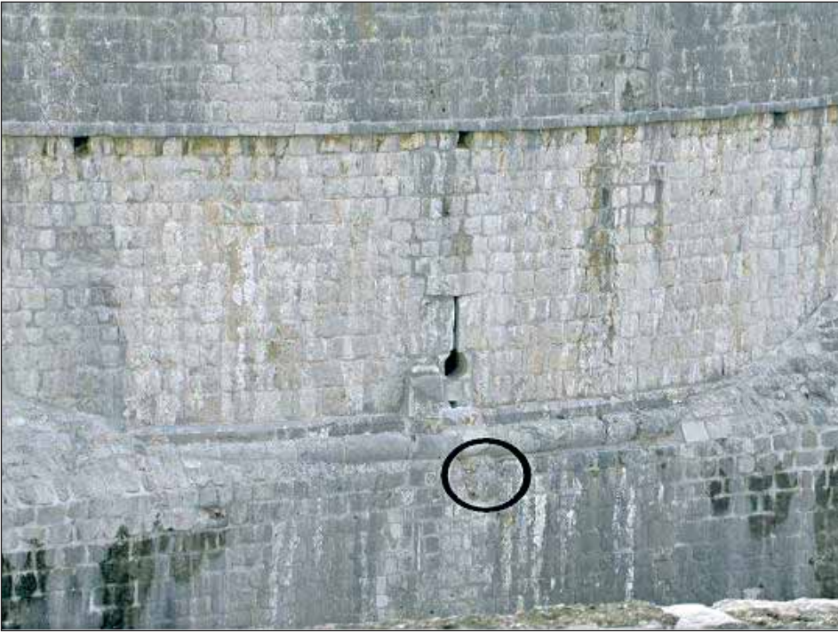
Figure 14: Minčeta Tower through which water was distributed to the City (the sealed opening)
