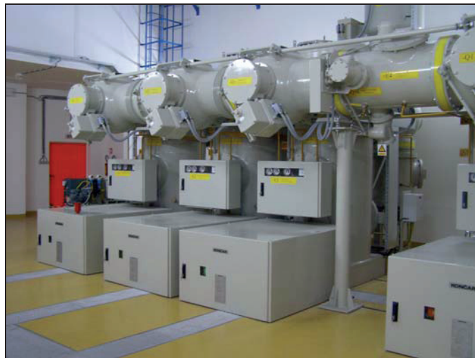
Fig. 2 View on one of the GIS 110 kV substation Dobri in which EMC conditions have been investigated
