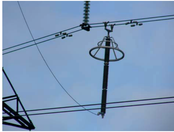
Figure 6. 400 kV line arrester in bottom phase.
