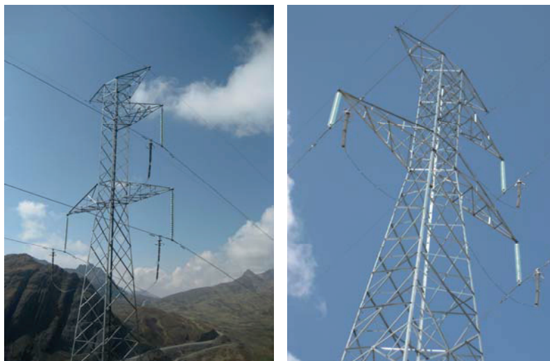
Figure 3 – Class 2 TLA with rated voltage of 192 kV installed along 220 kV line
