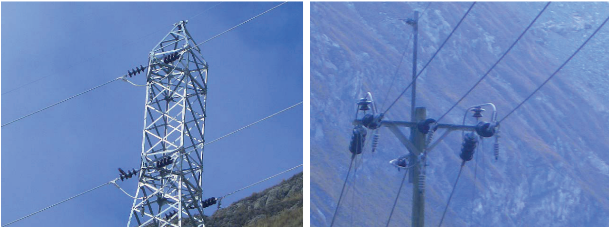
Figure 2 – Class 2 arresters installed on 23 kV overhead shielded distribution network
