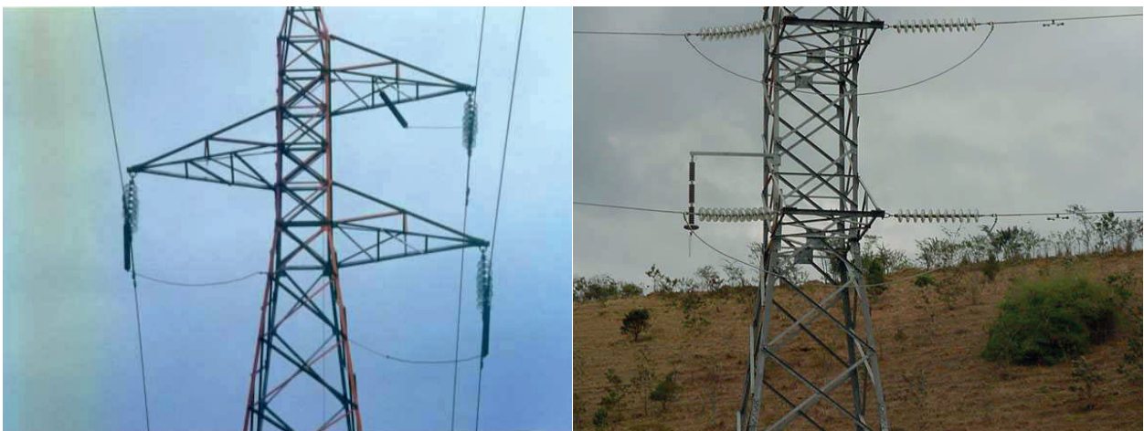
Figure 4 – Line arresters installed on 138 kV lines: Left – CEMIG / Right - UTEJF
