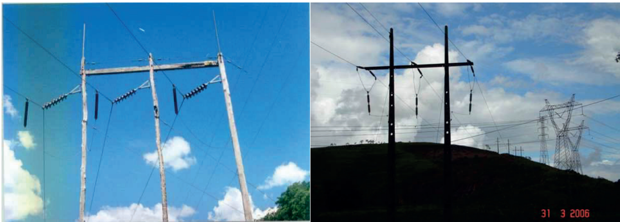
Figure 3 – Line arresters installed on 69 kV lines: Left CEMIG / Right Ampla
