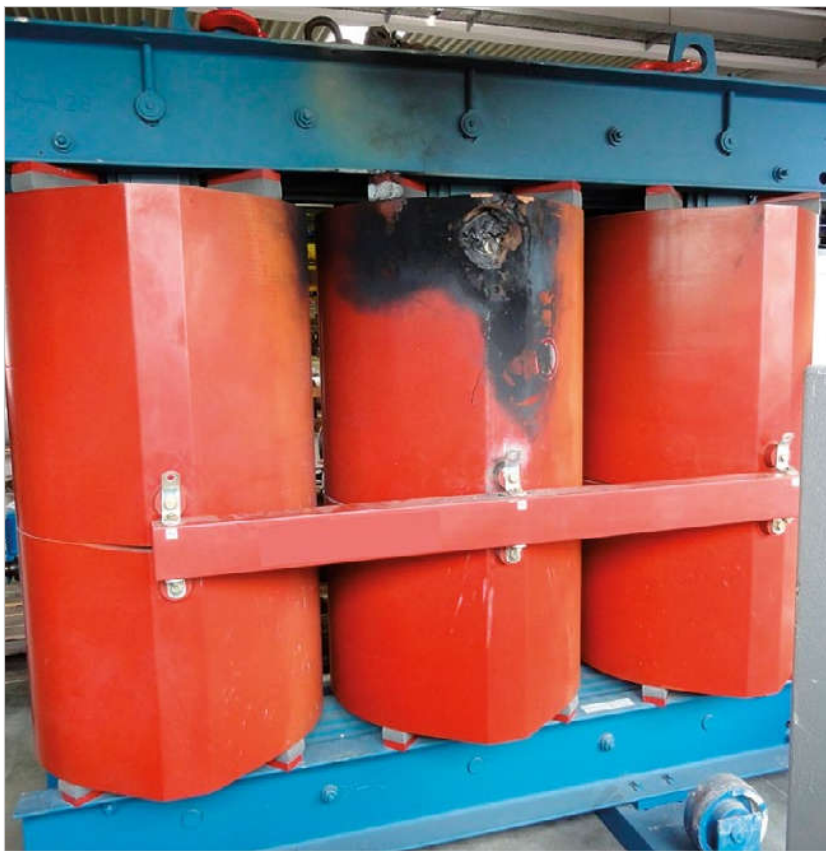
Figure 7. Breakdown fault on cast-resin transformer
