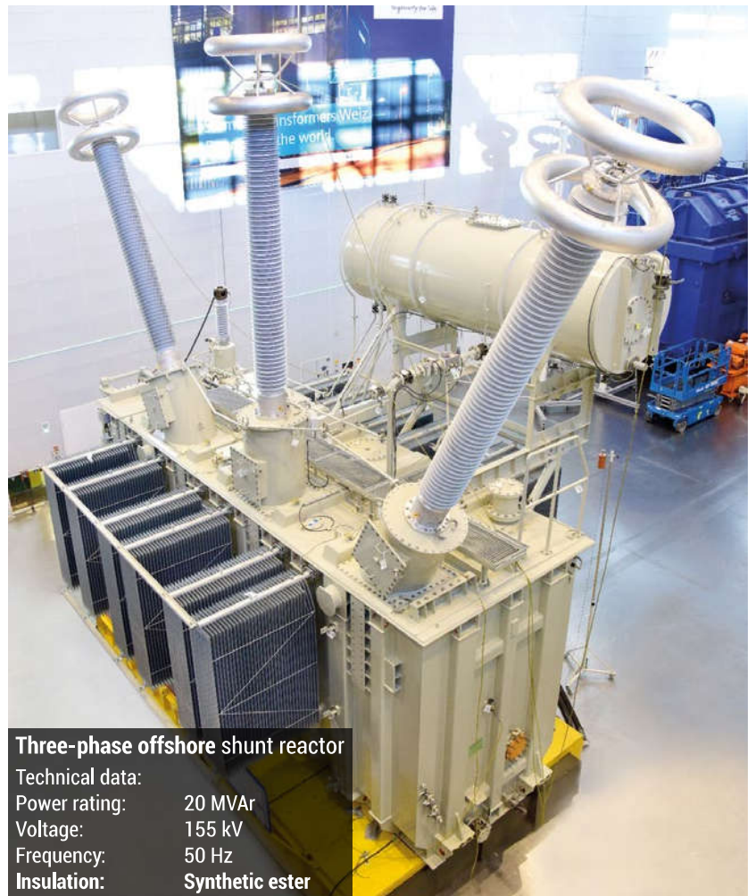
First shunt reactor with ester fluid
