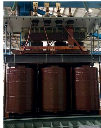
Figure 5 – RDT after short circuit test
