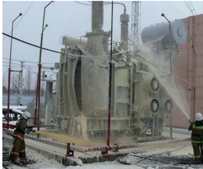
Figure 4 – Transformer in Western Siberia Substation after explosion
