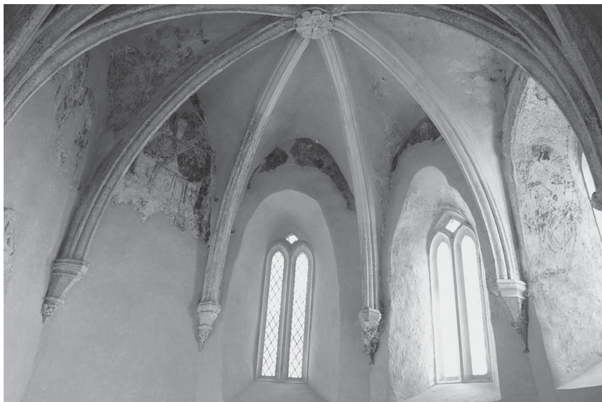
25. Unutrašnjost, pogled na ostatke gotičkih zidnih slika i prozore zaključka svetišta / Interior, view of the remains of Gothic wall paintings and windows in the sanctuary
