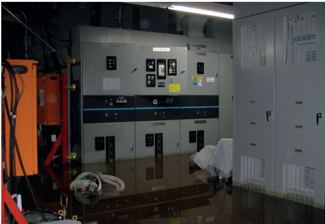
Figure 1 Example of Flood in Electric Equipment Room of Unit 6, pictured on 03.17.2011. (Source: TEPCO photo.tepco.co.jp/en/date/2011/201108-e/110810-01e.html )
