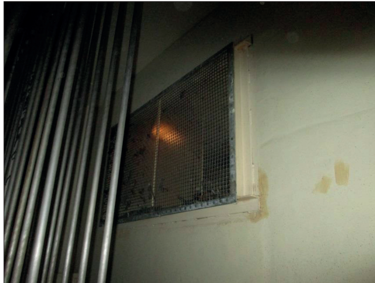
Figure 6: Reactor compartment ventilation entry
