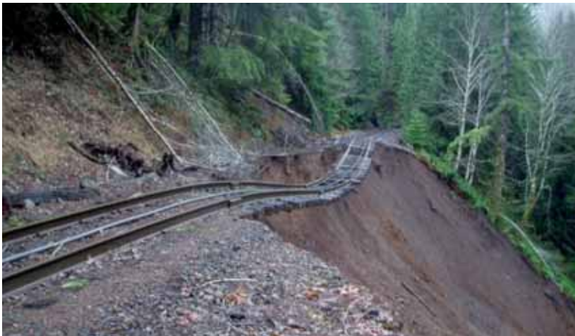
Figure 4. The impact of landslides onto the railway [1]
