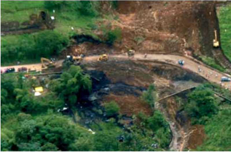
Figure 2. Landslide impact on Trans-Ecuador pipeline [13]
