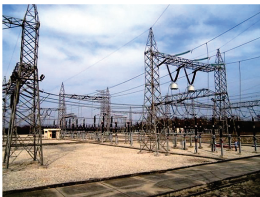
Figure 1 220 kV circuit in the Nueva Barranquilla substation. Source: Authors.
