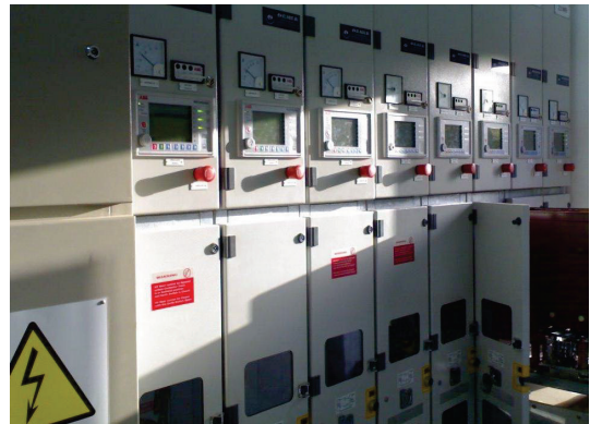
Figure 4 High voltage cells of engine
