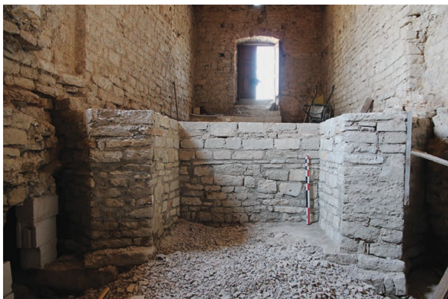
Fig. 37. Reconstruction of walls W 25, W 44, W 45 and partly W 65 during the restoration campaign (A. Milošević).
