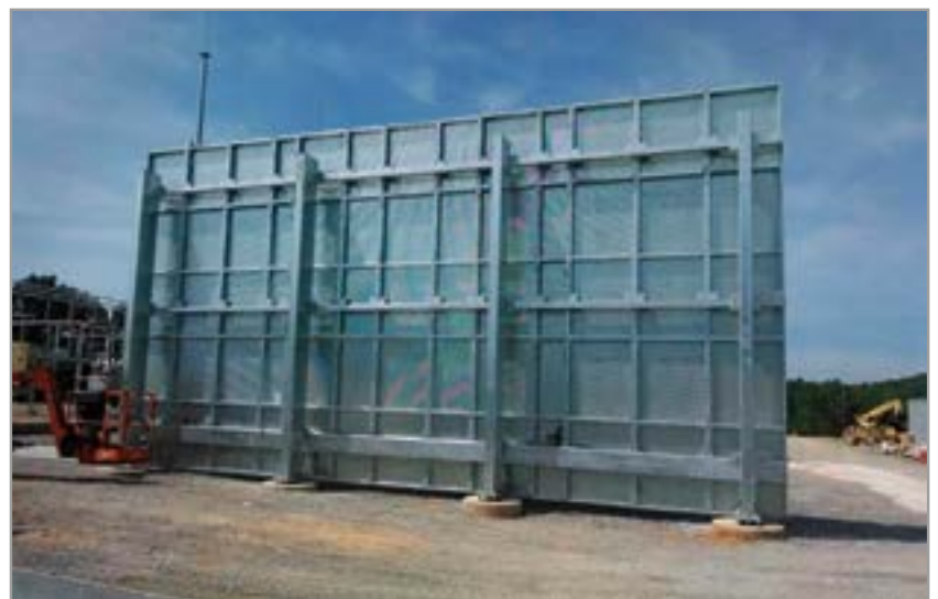
Figure 10. Modular steel fire and impact rated transformer barrier
