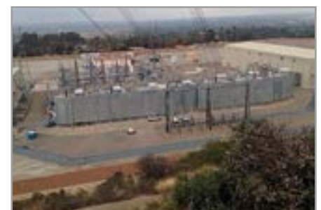
Figure 6. Major US substation protected from hillside by UL 752 Level 8 [2] ballistic fire barriers installed to NFPA 851 [1]
