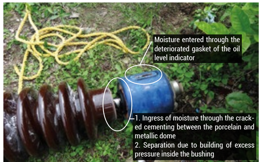
Figure 5a. The failed 245 kV, 1250 A OIP bushing showing cracked and separated oil expansion metallic chamber/dome from the porcelain insulator
