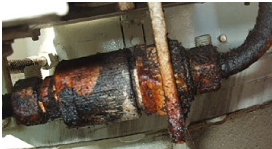
Figure 4. Rusty and leaking valve on CTG bushing
