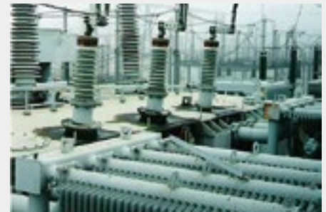
Figure 2. Oil leaks at the base flange of high voltage bushing pockets
