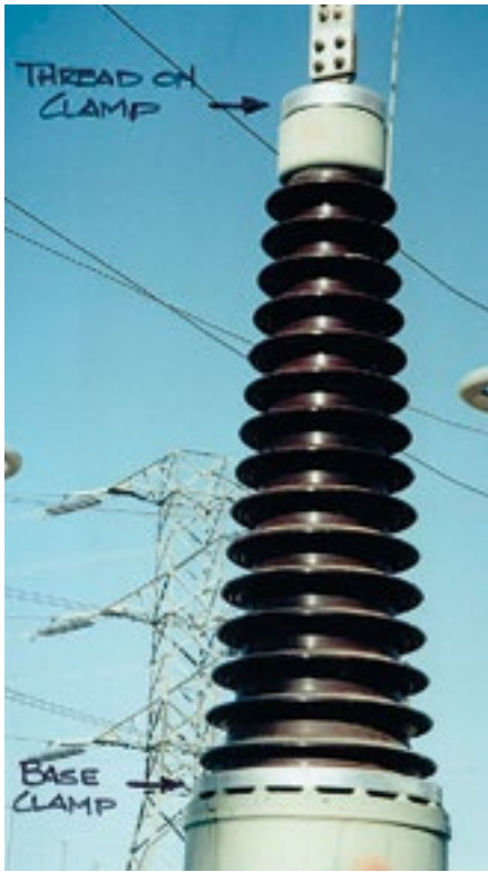
Figure 13. High voltage bushing with a precision aluminum split style clamp at the base as well as a threaded style clamp at the top of the bushing
