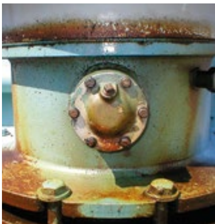
Figure 7. High voltage bushing leaking at the interface between the porcelain and the steel base
