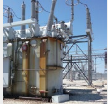
Figure 1. Unsightly oil leaks running down the side of a large power transformer
