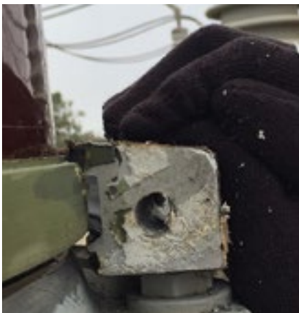
Figures 15a, 15b and 15c. Three views of a bushing with a portion of a previously installed bolted clamp removed
