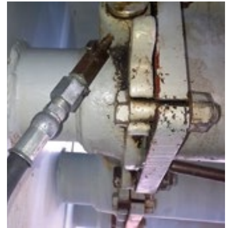
Figure 5c. An injection valve with the hose to the injection tool connected
