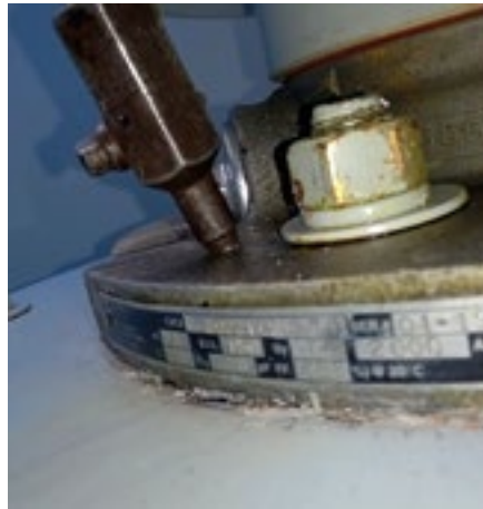
Figure 5b. Actual injection valve in place
