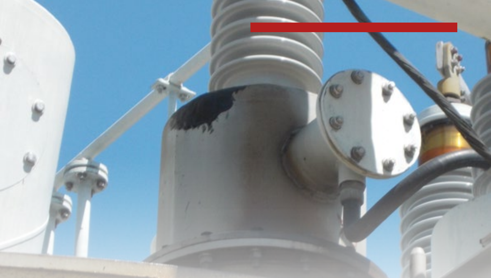
Figure 6. High voltage bushing pocket with oil stains running from the transformer top down the side. Note the black material at the top of the pocket, which is most likely an attempt by the utility to stop the leak with an externally applied material.
