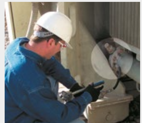
Figure 4. Repair being made to a lower level radiator flange by injecting sealant into the gasket groove with the transformer in normal service
