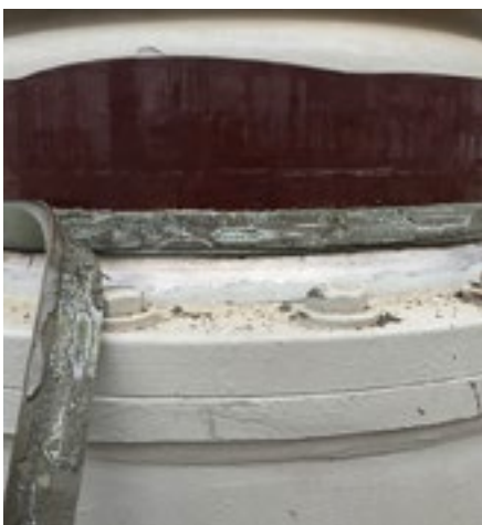
Figure 15d. Sealing compound cut away from the bushing
