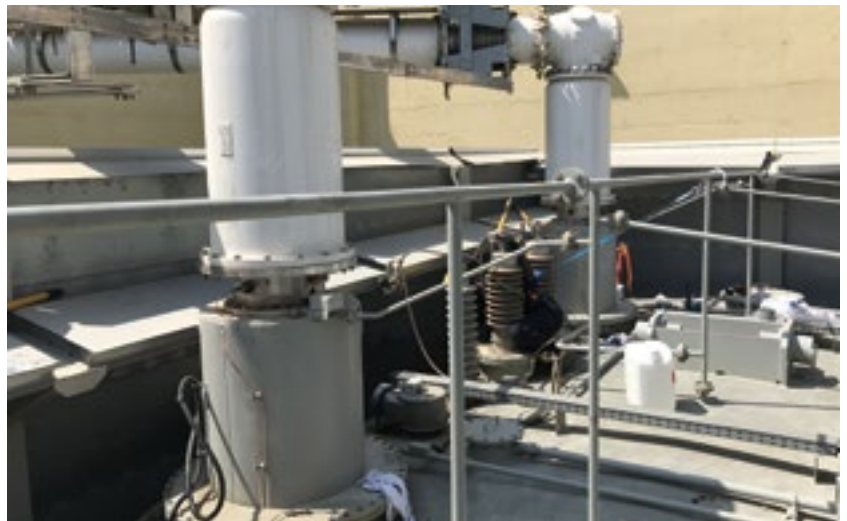
Figure 14a. SF 6 GIS bus connections to high voltage bushings on top of a transformer
