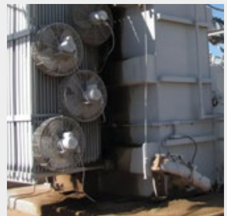
Figure 3. Oil leaks running down the side of a large power transformer and contained with oil absorbent material
