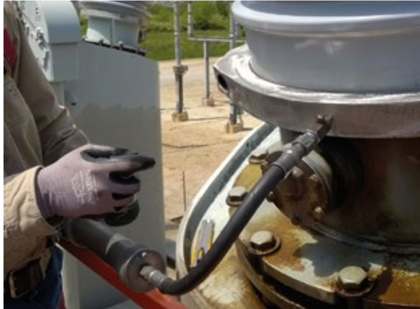
Figure 11. Technician pumping the leak seal compound into the clamp around the bushing
