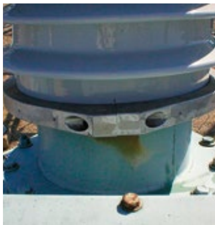
Figure 8. Close up of a precision fabricated aluminum clamp installed at the base of a high voltage bushing
