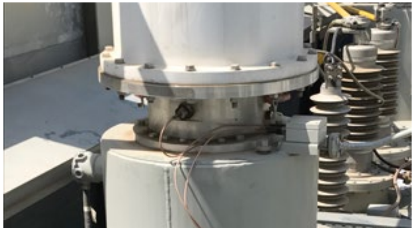
Figure 14b. Close up of the GIS to transformer connections
