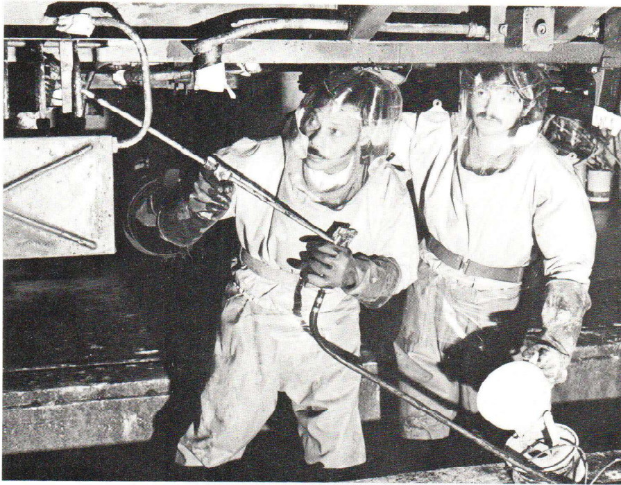
FIG. 4 – Equipment used for the removal of asbestos insulation. From British Rail rolling stock.
