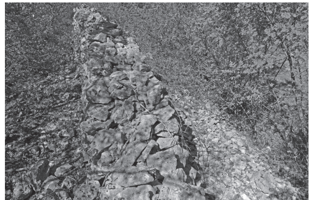
Figure 10. Dry-stone Wall on Top of the Piles of Rock (photo: N. Cesarik).
