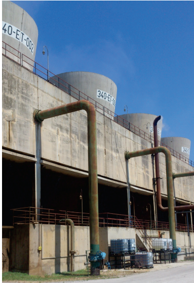
Figure 1 The cooling towers of the INA fuel refinery. At the forefront: water supply pipes and air intake.
