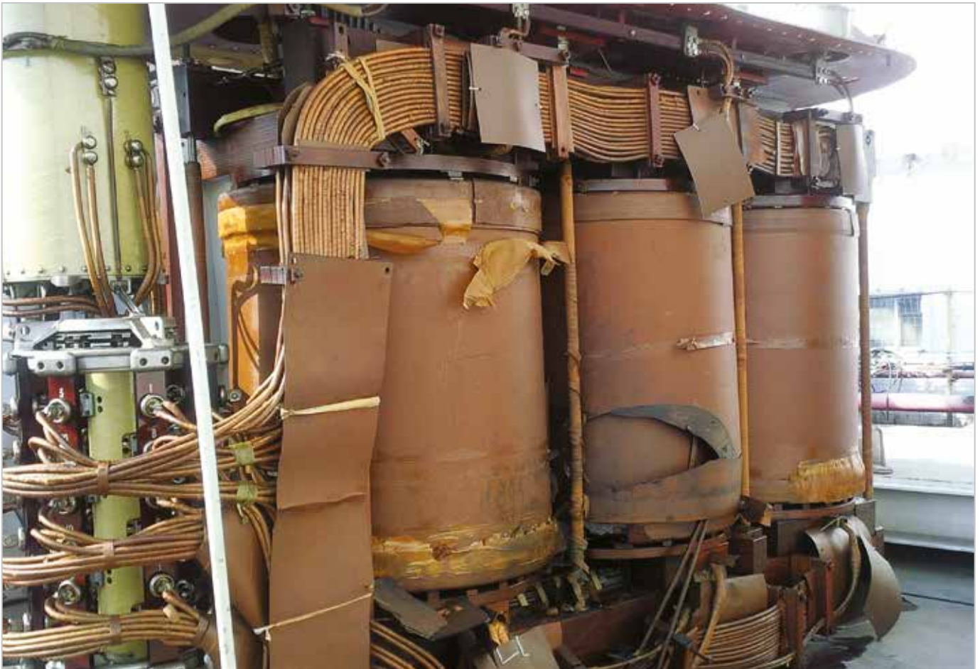
Figure 4. The failed transformer due to excessive moisture
